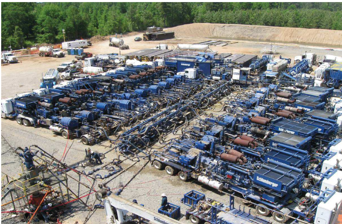
Figure 5-2. Hydraulic fracturing site showing equipment used on-site during the chemical mixing process.
